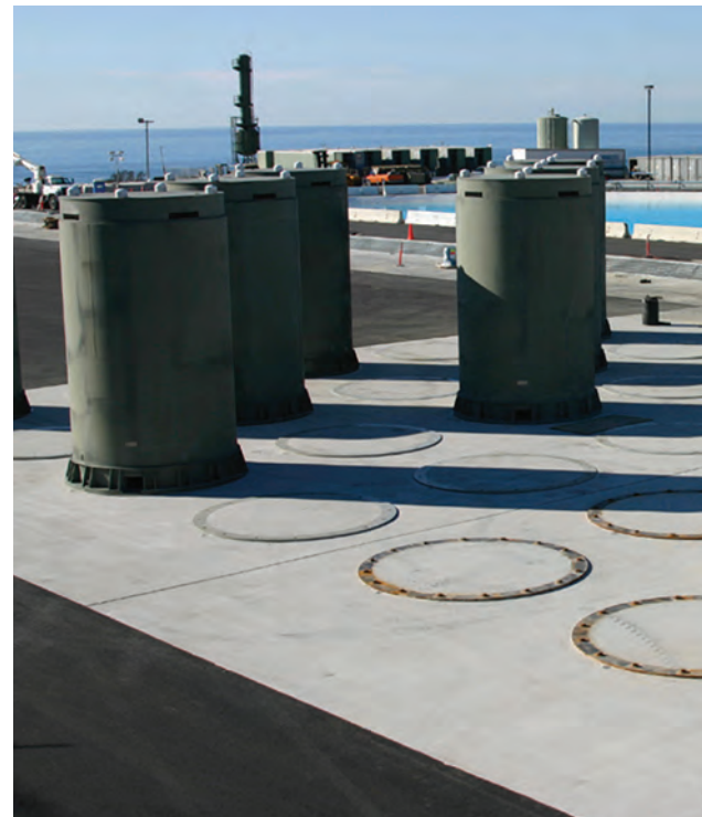
Dry casks at the Diablo Canyon Site near Avila Beach, California. Credit: The U.S. Nuclear Regulatory Commission.
